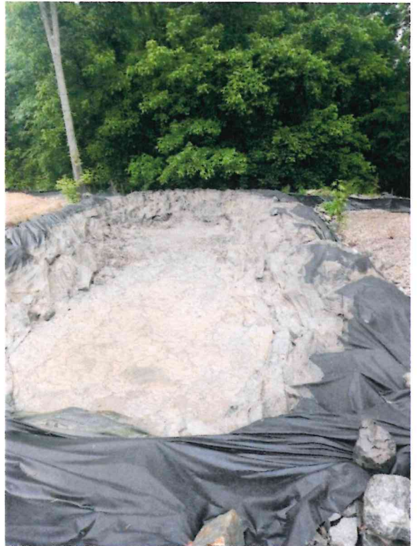
5/13/2024 - Inside of berm around MH 1750 before cleanup
