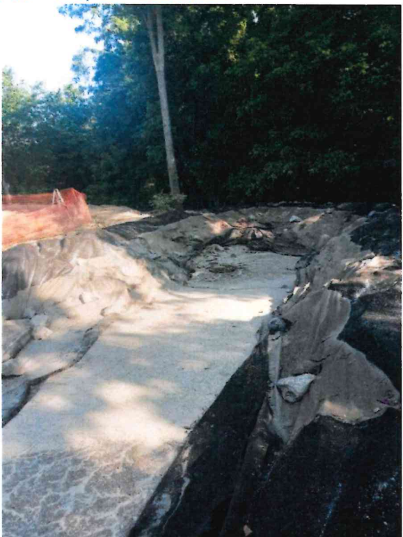
5/20/2024 Inside of berm around MH 1750 before cleanup
