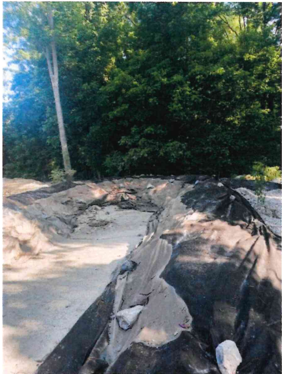
5/20/2024 Inside of berm around MH 1750 before cleanup
