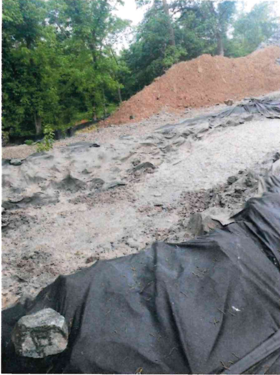
5/13/2024 - inside of berm around MH 1750 before cleanup
